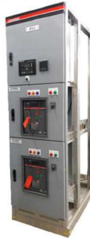
Automatic Transfer Switch
