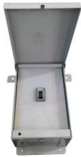
Enclosed Circuit Breaker
