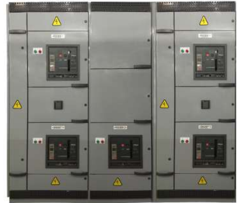
Low Voltage Switchgear
